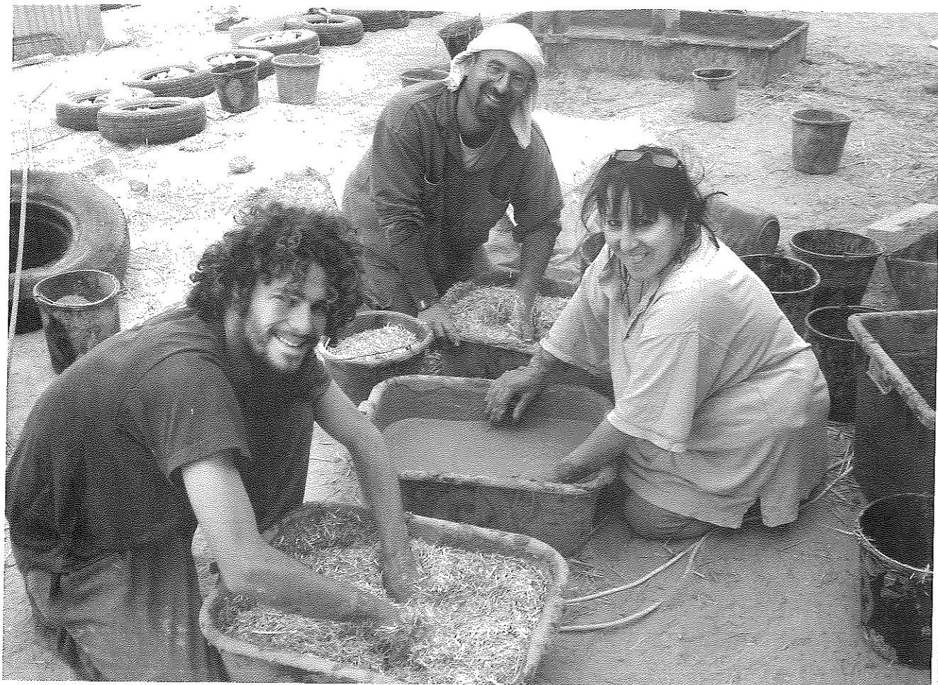
Mike (left) from Kibbutz Lotan, shows Bedouin villagers at Wadi el N'aam how to mix earthen plaster for the new clinic.
